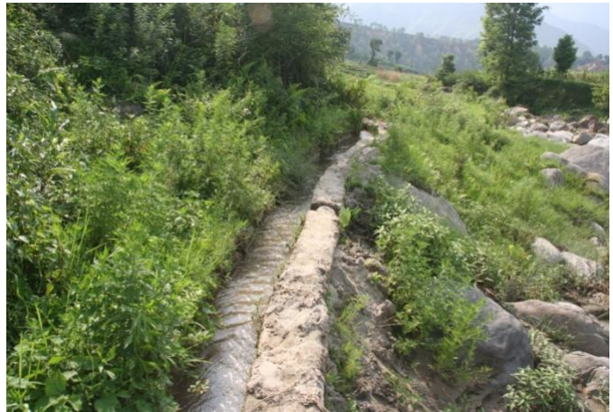
Poor infrastructure condition
