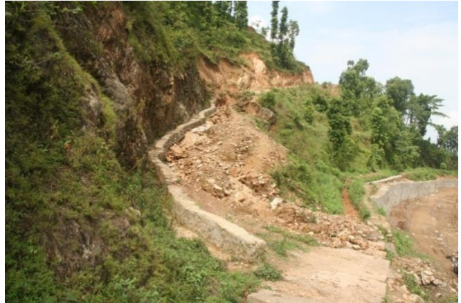
Earthquake damage on Kabilas-Simarai I.P, Chaugada V.D.C.
