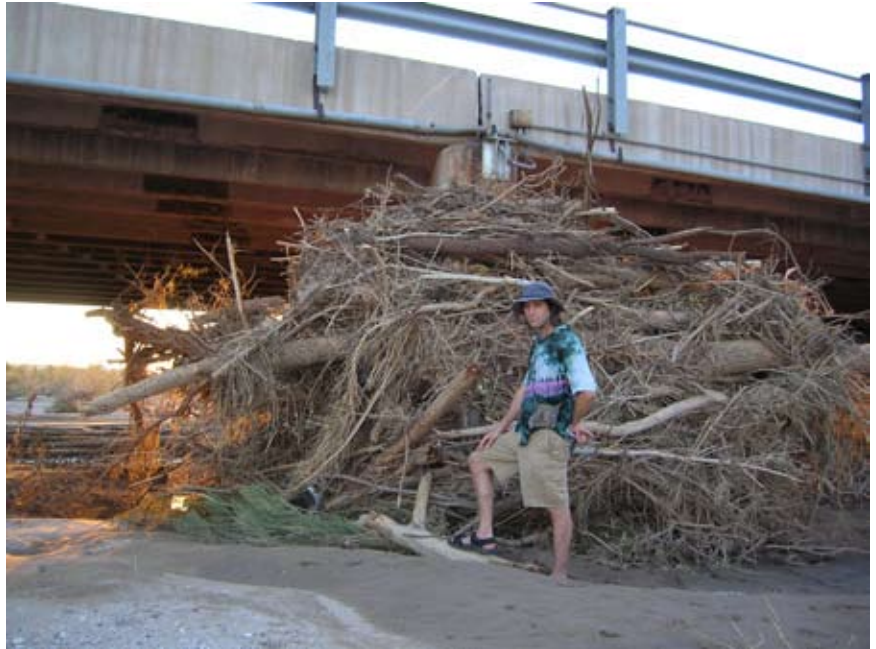
Figure 1. Tucson resident Robert Segal stands by debris collected by supports of the First Avenue bridge where it crosses the Rillito River. The July 31 high waters that carried the logs had moved downstream or underground by August 5, when this picture was taken.
