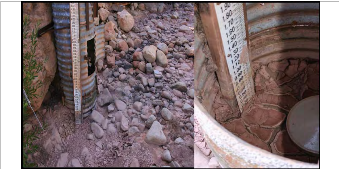
Figure 6.4. Accumulation of rock debris (outside) and sediment (inside) the stilling well in Captain Tom Wash. Both conditions would increase the stage height measured in this station.
