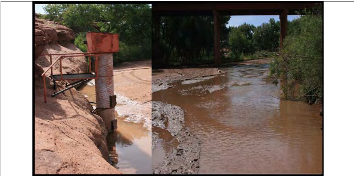
Figure 6.2. Two photographs showing opposite sides of Chinle Creek at Chinle stream gaging station. The stilling well is on the left while most of the flow occurs on the right side opposite the stilling well. The large amount of accumulated sediment is responsible for the situation.
