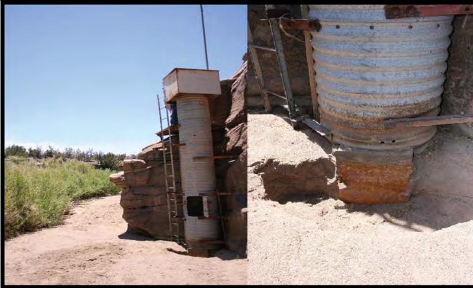
Figure 6.3. Deep sediment accumulation and vegetation growth in the gaging station at Black Creek .Note the depth of the accumulated sediment on the right hand side photograph.
