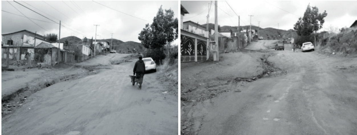
Figures 2-3a and 2-3b. Damage is evident on unpaved roads in a Nogales, Son., colonia after heavy rain (1/28/2010). Source: Photos by Jeremy Slack.
